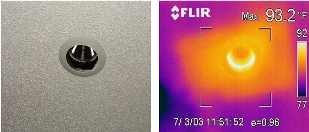
Figure 3. Ceiling penetration and insulation problem
