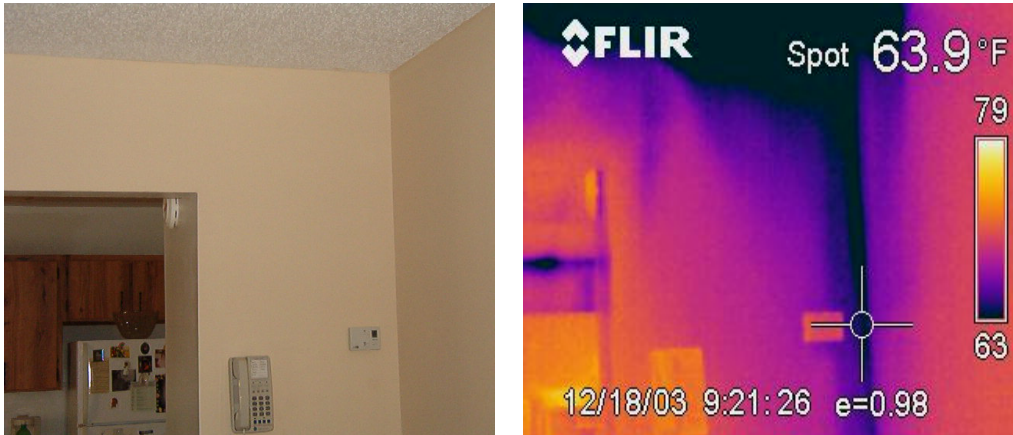
Figure 5. Cold air being drafted in a hollow wall behind the thermostat
