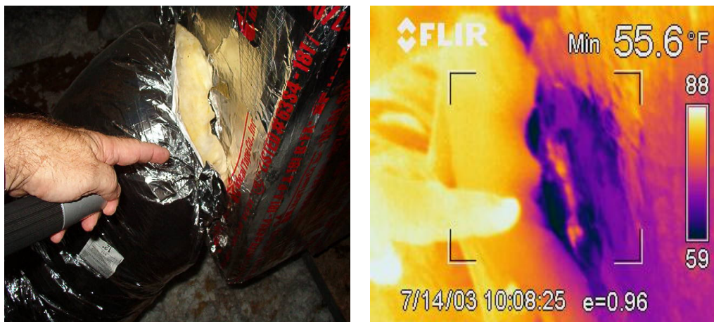
Figure 8. Supply junction of flex duct and disbursement box that was not sealed or taped
